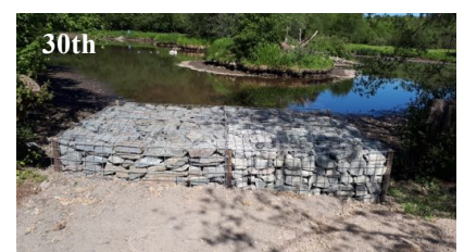
Raked out the excavated soil to restore the bank and fill in around the platform.
