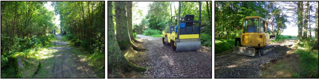
Day 6. Final section of path through the wood was already covered with terram and thin layer of type 1. More type 1 was added to cover tree roots and rolled. Soft area near field gate left to dig out, lay terram and fill with stone and type 1.
