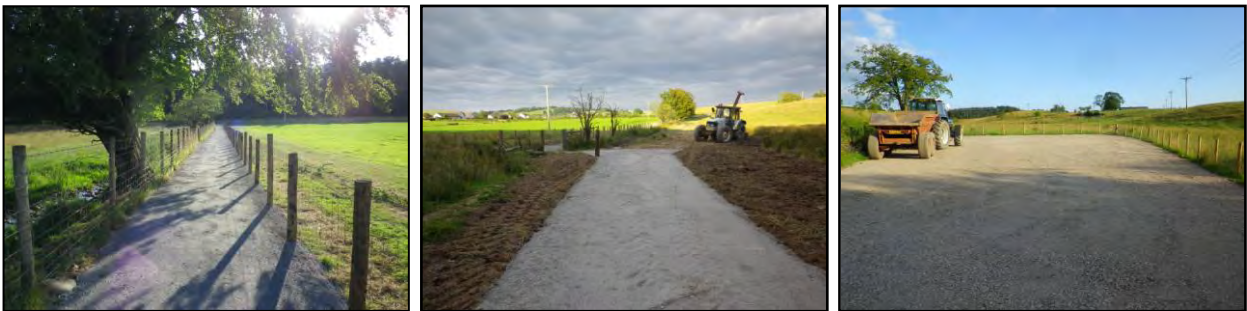
Day 8. Lower section of field path fenced. Hunting gate to Wood gate surfaced with type 1 and dust. Bottom end of field ditch dug out as far as pipe and area of field around Wood gate tidied. Remaining type 1 spread evenly over car park area.
