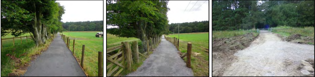
Day 7. Whole length of field path covered with dust and further rolled. The fencers start on the middle field section of the path. The section between from the Hunting gate to the Wood gate filled with stone and type 1.
