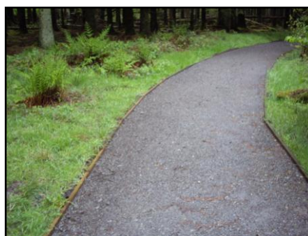
26th April -S1 Environmental Studies class fitted new boards along the Reserve path to replace the old, rotten boards.
